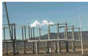
The result of a failed breaker
